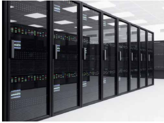
Data center | E-bus charger
